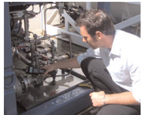
GasCheck 5000is being used to leak test machinery at PSL Energy Services, Singapore
